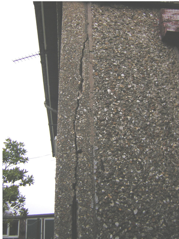
Photograph 2 – Vertical Cracking Of Corner Post
