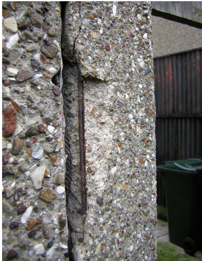
Photograph 3 – Spalling Of Corner Post
